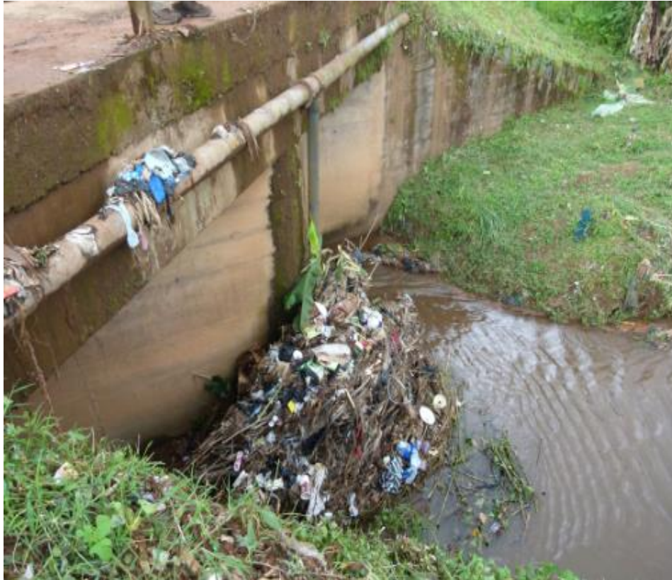
Figure 2. River with garbage dumped into it.
